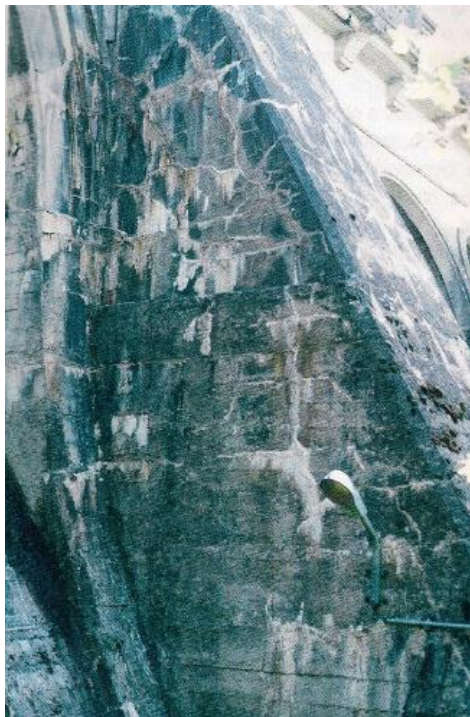
Fig. 4.8 - Surface map cracking on a dam concrete buttress with gel exudation and staining
