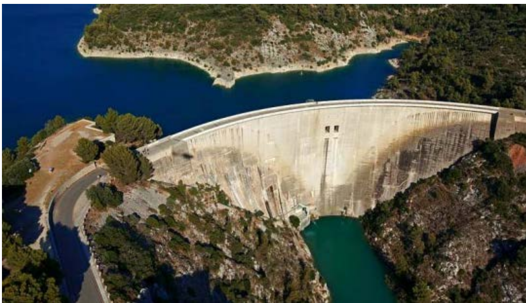
Fig. 3.9 – Bimont dam affected by DEF [3.19]
