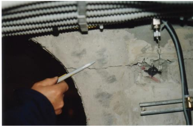
Fig. 4.11 - Particular of the structural crack in the upper gallery
