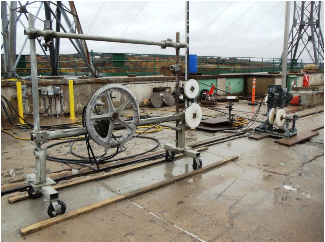
Cover photograph: Diamond wire saw cutting equipment in use re-cutting slots in the gravity dam intake at Mactaquac Generating Station, New Brunswick, Canada, 2011
