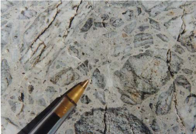
Fig. 4.15 - Cracks partially filled with silica gel in a dam concrete core.
