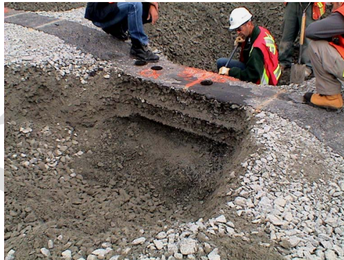
Figure 4.2 Test field for an asphalt concrete core after removing the filter zone (Nemiscau 1 dam, Canada)
