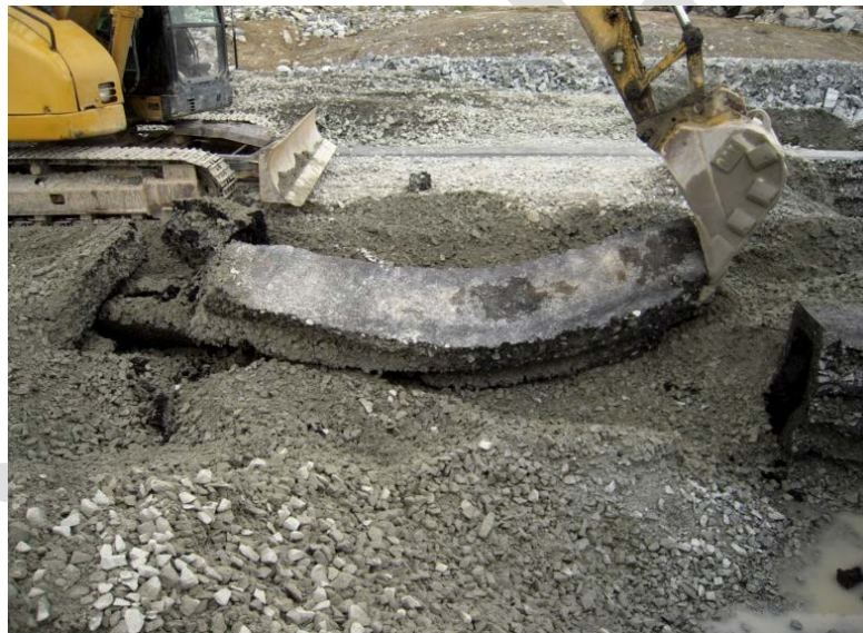
Figure 4.6 Asphalt concrete cores are very flexible and ductile (Trial test at Nemiscau 1 dam, Canada)
