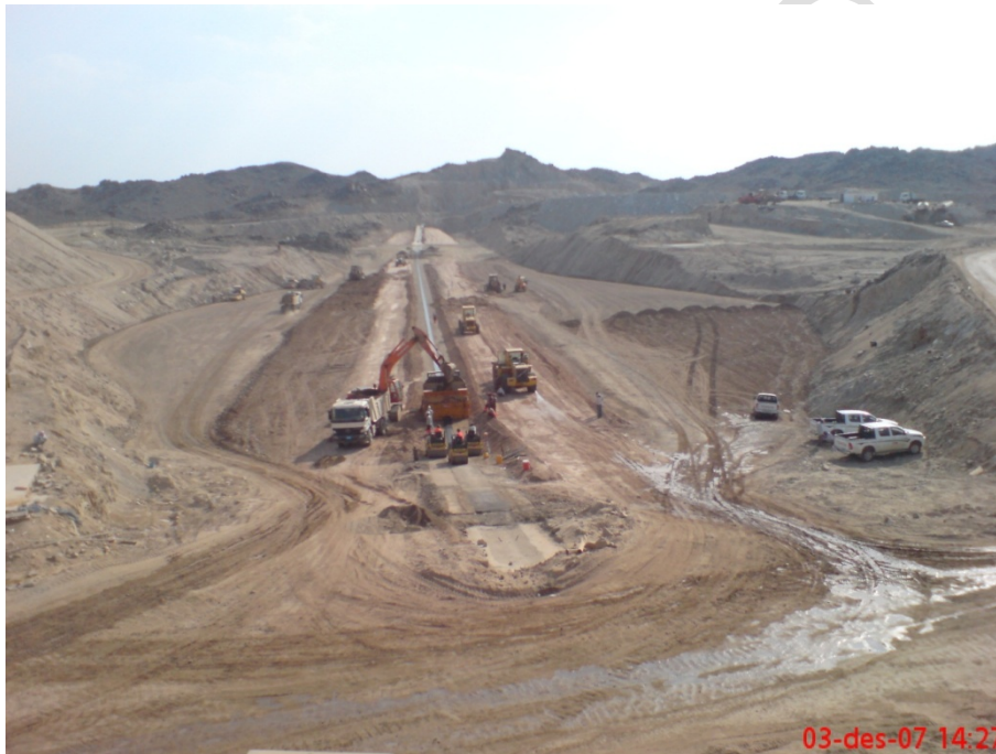
Figure 3.3 Murwani Dam, Saudi Arabia, very hot climate conditions
