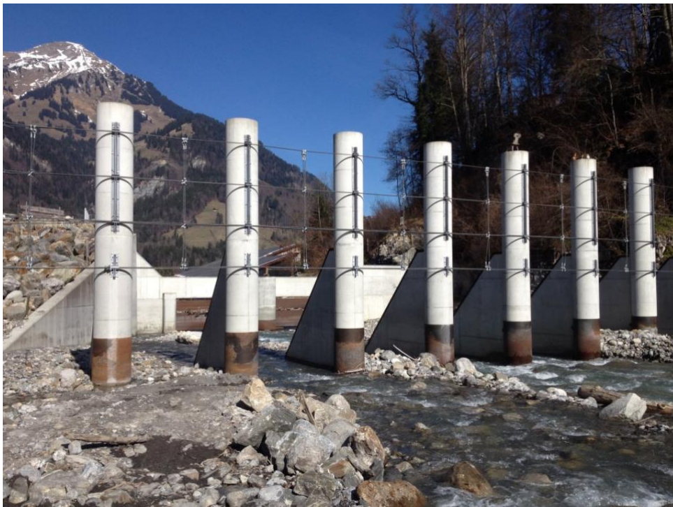
Fig. 4.10 Large wood and trash cable racks installed on the Chiene river, Canton Bern (Photo: Emch + Berger AG), Boes et al. (2017)
