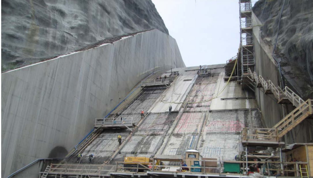
Figure 3.7 Sectioned spillway works to ensure “return to service” with “t” days of notice (courtesy of BC Hydro)
