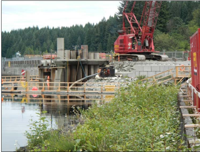
Figure 3.4 Temporary upstream cofferdam to protect low level modification works (courtesy of BC Hydro)
