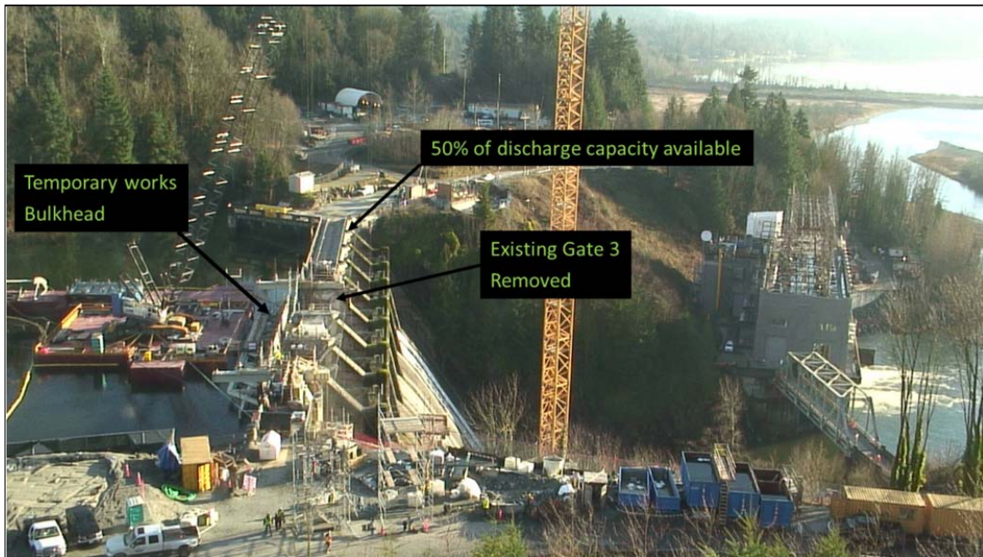
Figure 3.5 Partitioning of spillway discharge function during spillway modification (courtesy of BC Hydro)
