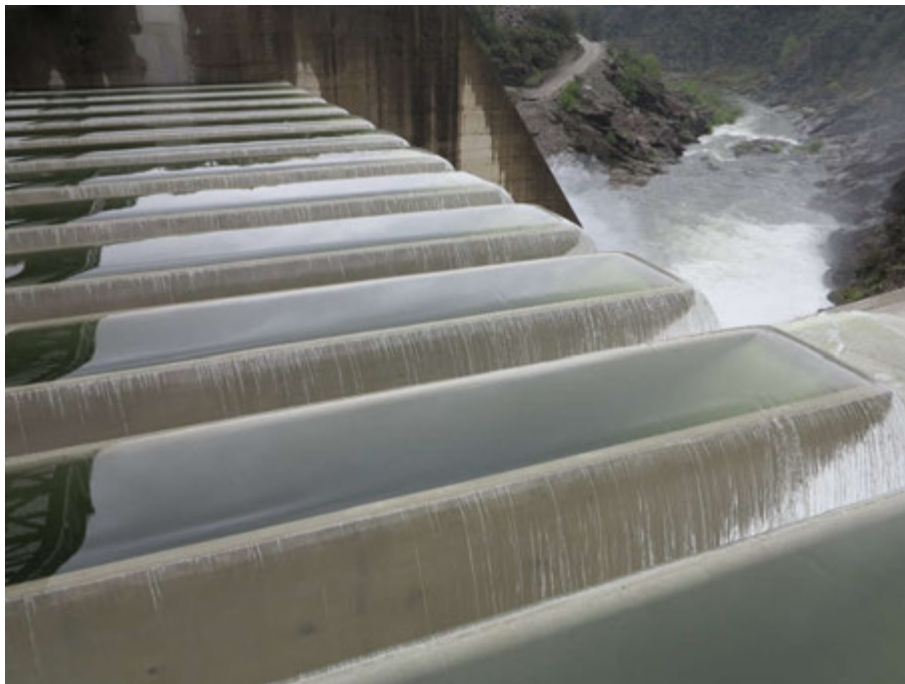
Figure 6.7 - Flow over the Malarce dam PKW (France) with an upstream head of a few cm (Photo courtesy of EDF)
