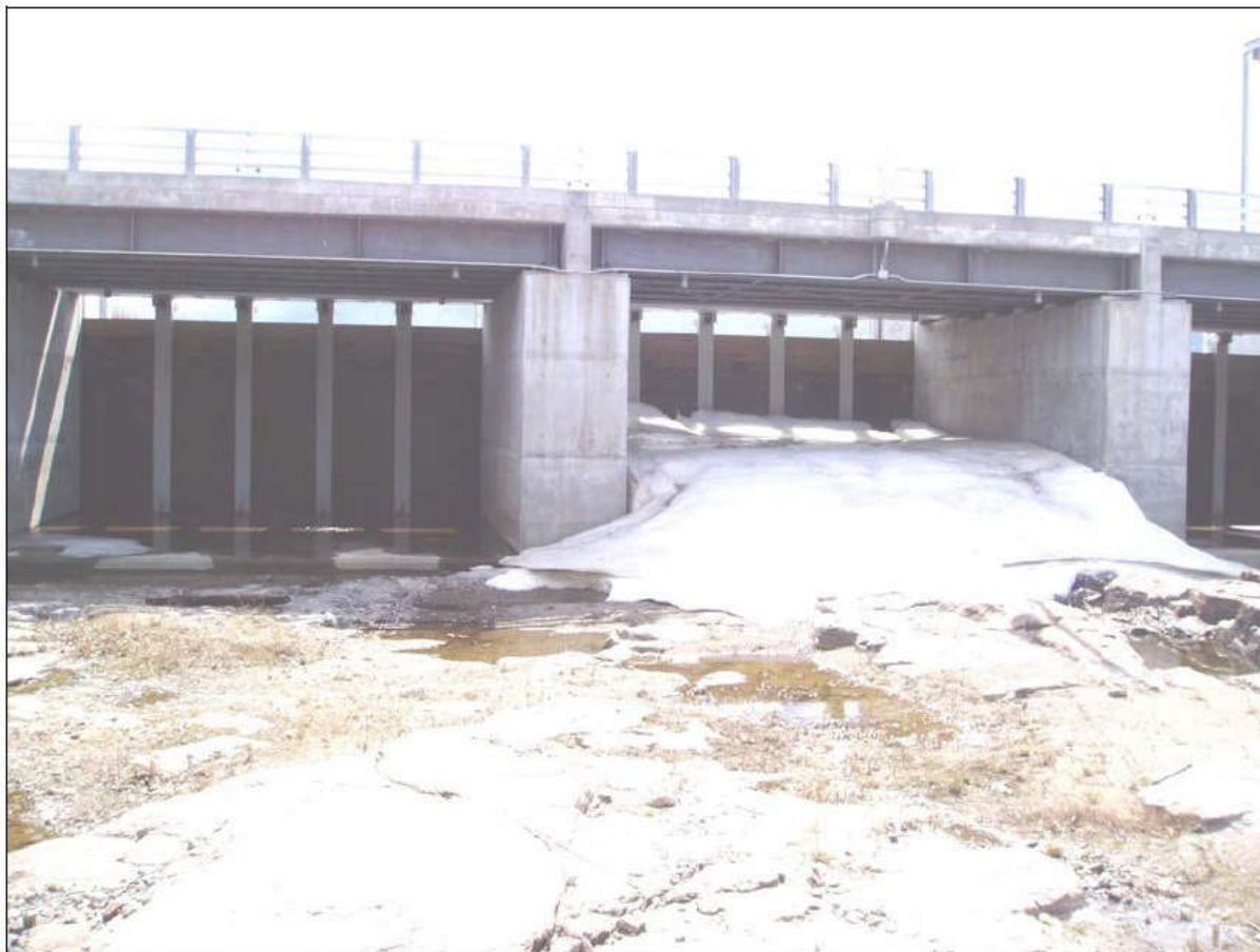
Fig. 8.4 - Pont Arnaud: Gate leakage in winter creating aufeis (ice accumulation) and reducing significantly the spillway capacity (Hydro-Québec).
