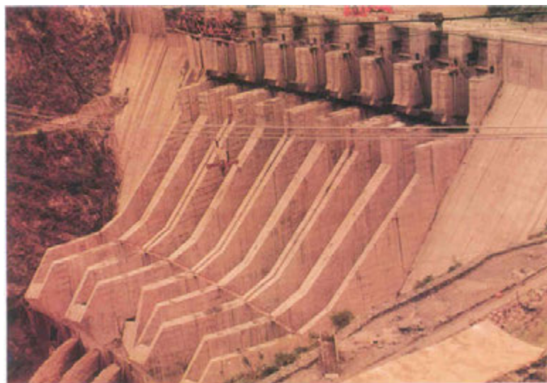
Fig. 2.9 – Orifice and bottom outlets of the spillway of Chamara I Project, in India
