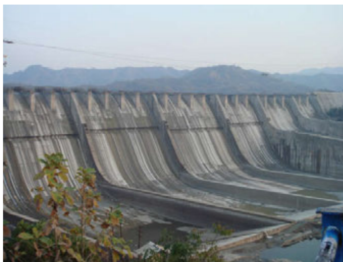
Fig. 2.12 – Sardar-Sarovar 87 000 m 3 /s spillway in India (piers and radial gates not yet installed)
