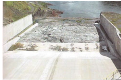
(b) Extended lining after erosion tests
