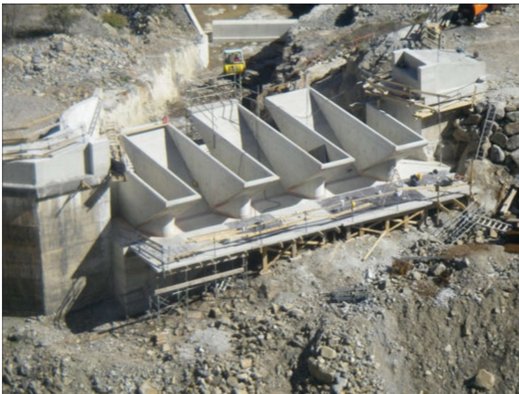
Figure 6.1 - View of the PKW spillway of Gloriettes Dam in France during construction
