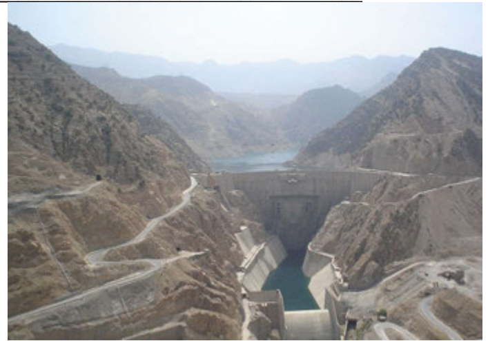
Left: Plunge pool lining under construction Above: View of the completed works
