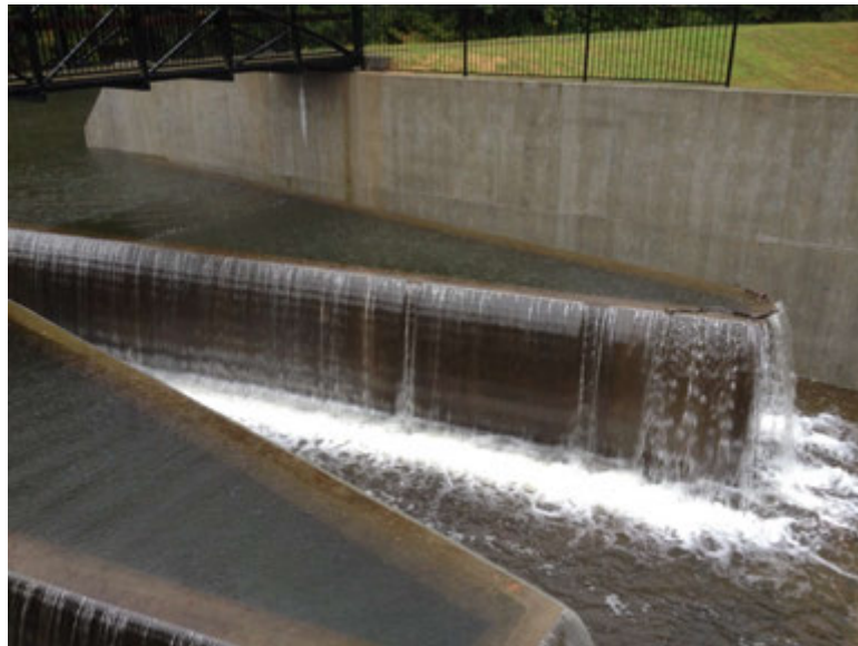
Figure 5.7 - Nappe vibration (photo courtesy of Schnabel Engineering, USA)
