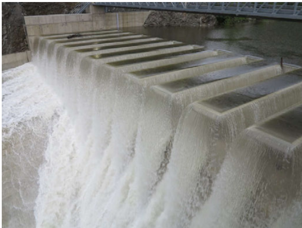
Figure 6.2 - View of the PKW spillway of Malarce Dam in France during spillage (Photo courtesy of EDF)
