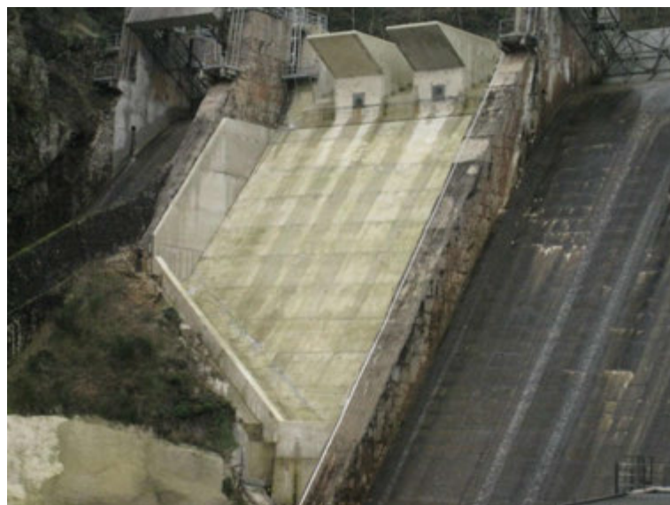
Figure 6.10 - Smooth spillway and inclined flip bucket downstream of the Saint Marc dam PKW
