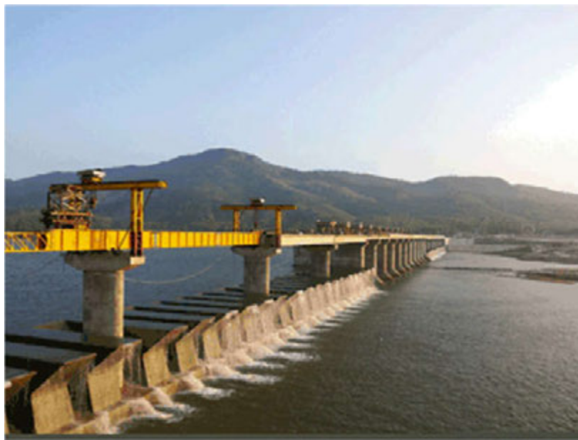
Figure 6.14 - The Van Phong barrage in Vietnam (Courtesy of M. Ho Ta Khanh)
