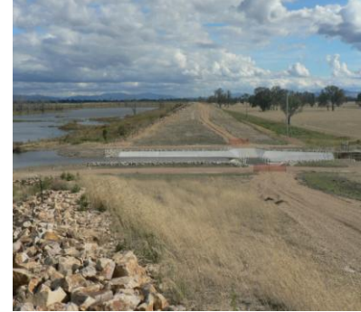
Embankment Breach and Wetland and showing overflow control structure
