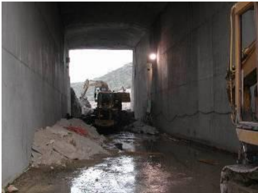
Fig. 7 – Civil works (in progress) to channel the water through the buttresses of the vault to be demolished
