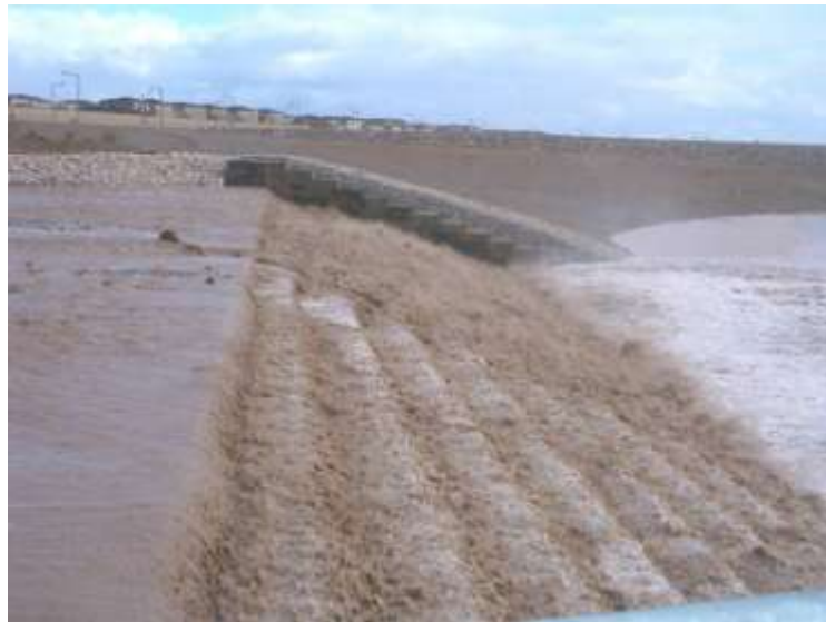
Photograph 7.8: 2004 storm overview at Red Rock Detention Basin spillway (Abdo and Adaska, 2007)
