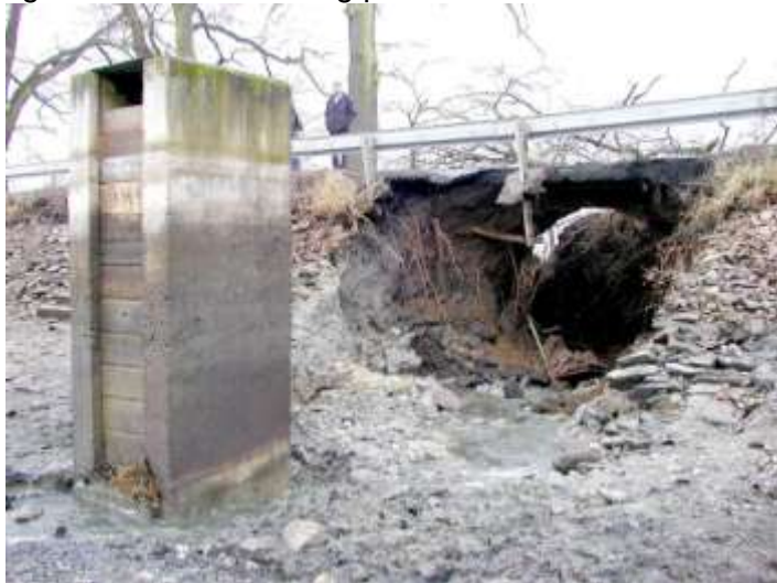
Fig. 3.6 - Cavern in the dam body as a result of wooden bottom outlet decay and internal erosion (Czech Republic)
