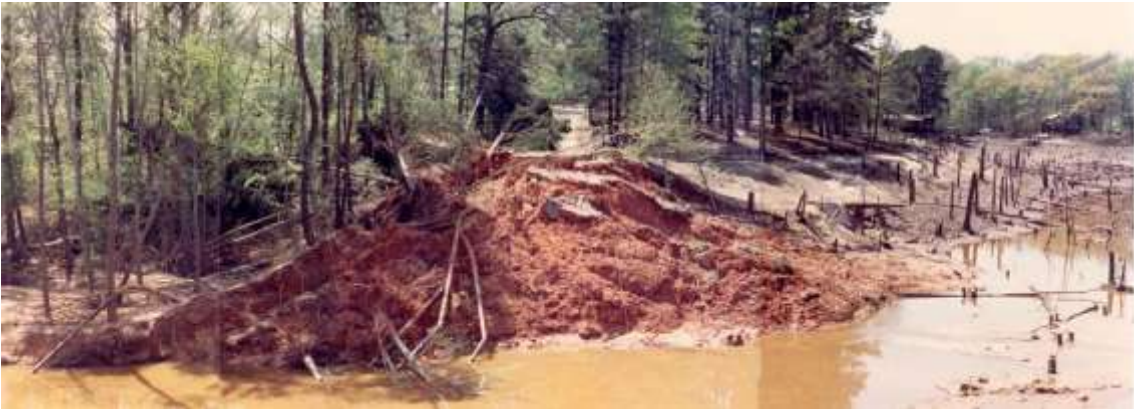
Fig. 3.4 –Nix Lake dam failure in Texas, in 1989 (ASDSO, 2007).
