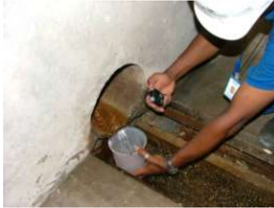
Fig. 6.1 – Leakage measurement using a vessel and a chronometer.
