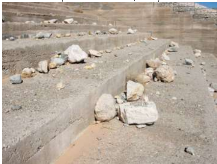
Photograph 7.9: Boulders deposited on the RCC steps during 2005 storm (Abdo and Adaska, 2007)
