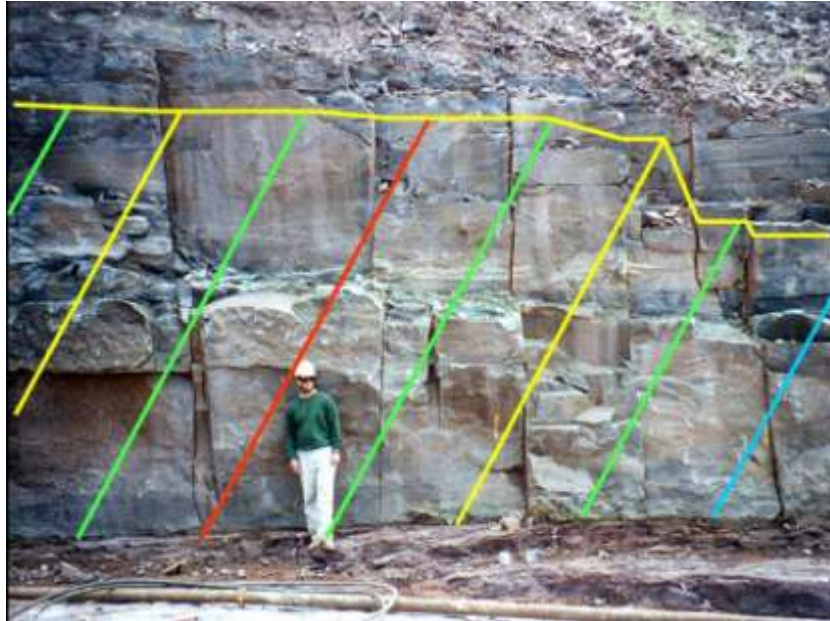
Photograph 7.10: Vertical rock joints shown with angled grout hole orientation (Penn Forrest Dam Rehabilitation, USA)
