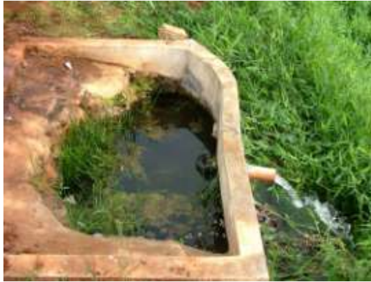
Fig. 6.3 – Vegetation debris upstream the weir gauge.
