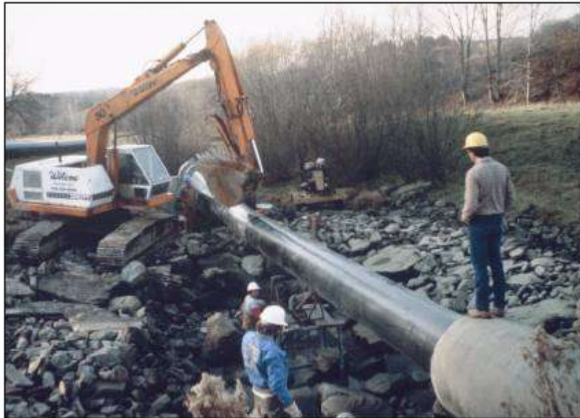
Photograph 7.15: Example of sliplining – insertion of plastic (high density polyethylene) pipe into larger diameter concrete pipe (from FEMA, 2005)
