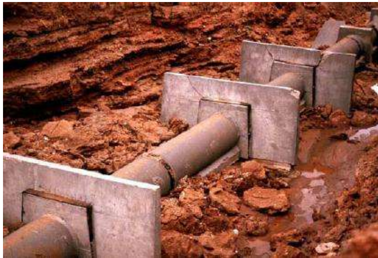
Fig. 5.5 – Pipe with intact anti-seepage collars shortly after failure of a small dam (McCook/2004).
