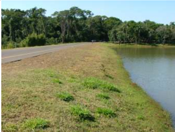
Fig.5.14: Upstream slope protection with grass at the Chibarro dam, 12 m high, in Brazil (fetch = 300 m).
