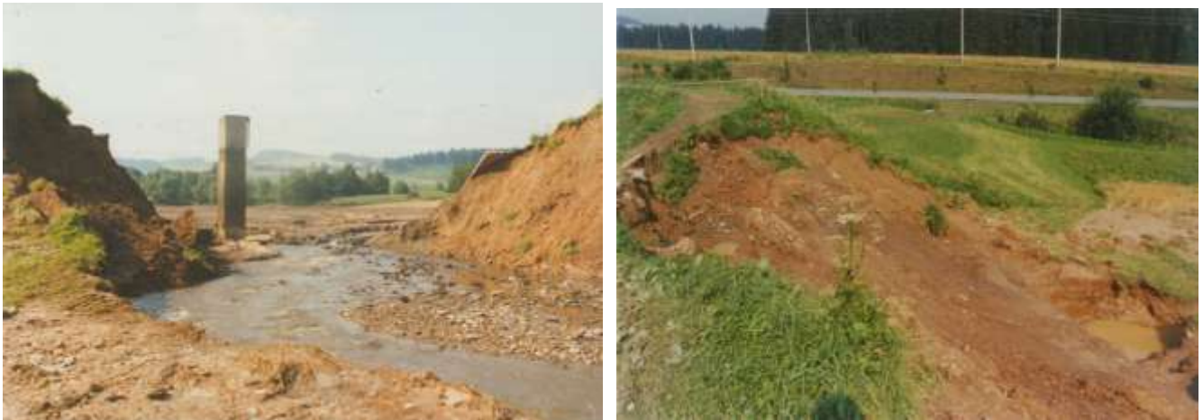
Fig. 4.1 - Busek pond in Czech Republic – dam break after overtopping in August 1991 (extreme summer raining) [2].
