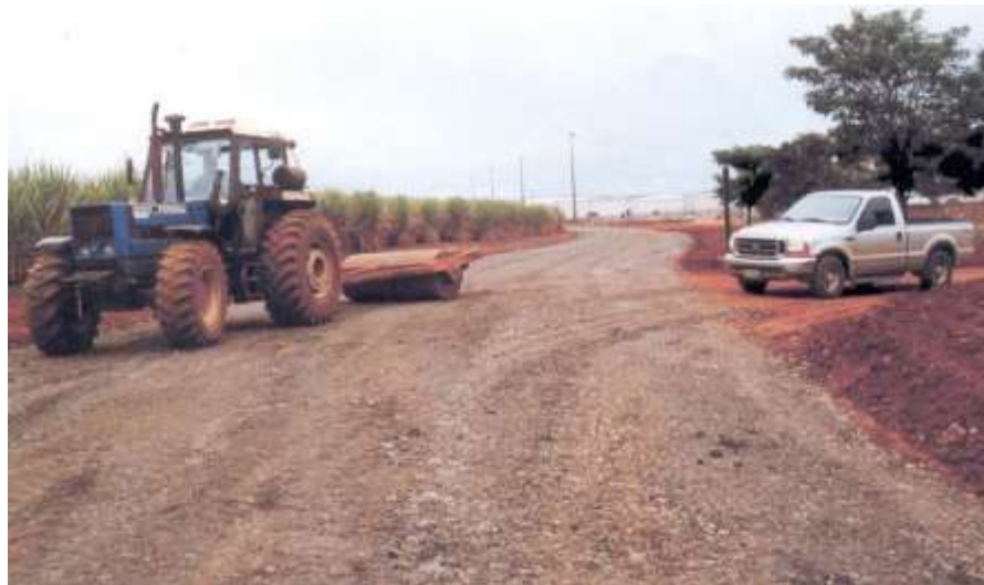
Figure 5.17: Constructing a rural road using a granular material composed by gneiss, limestone and bituminous shale.
