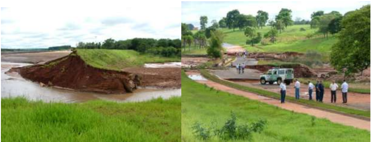
(A) (B) Fig. 3.3 – (A) Paraguaçu embankment dam failure by overtopping, after severe flooding in Brazil. (B) Downstream erosion damages at an embankment road access, in January, 2007.
