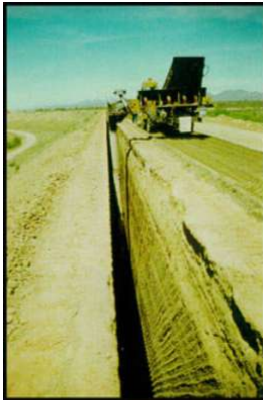
Photograph 7.14: Central sand filter installed by open trenching from the crest of an existing low-height flood control dam in southwestern USA
