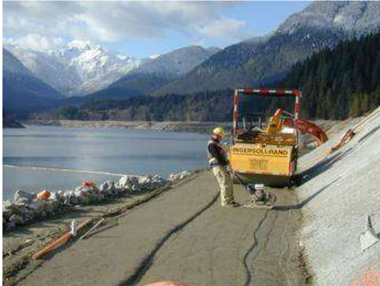
Photograph 7.12: Construction of a roller-compacted concrete (RCC) blanket extension in the abutment of Cleveland Dam, near Vancouver, Canada. The base of the RCC blanket was tied into a vertical plastic concrete seepage cutoff wall (Singh, et al., 2005) (image from www.waterpowermagazine.com/story.asp?storyCode=2033046 ).
