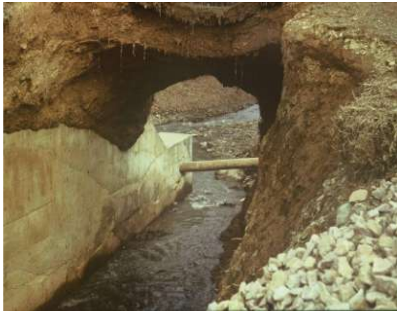
Fig. 3.8 – Earth Internal erosion after earth frost penetration along spillway concrete wall
