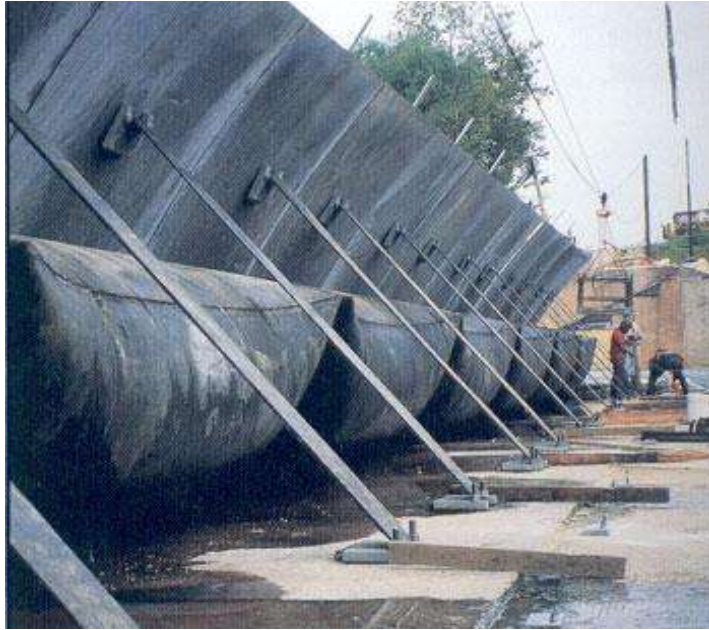
Photo.2.19 Spillway gates with inflatable air bladders
