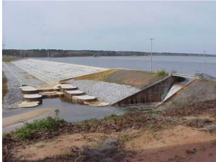
Photograph 7.6: A view of principal and auxiliary spillways at Lake Tholocco Dam (Abdo and Adaska/07)
