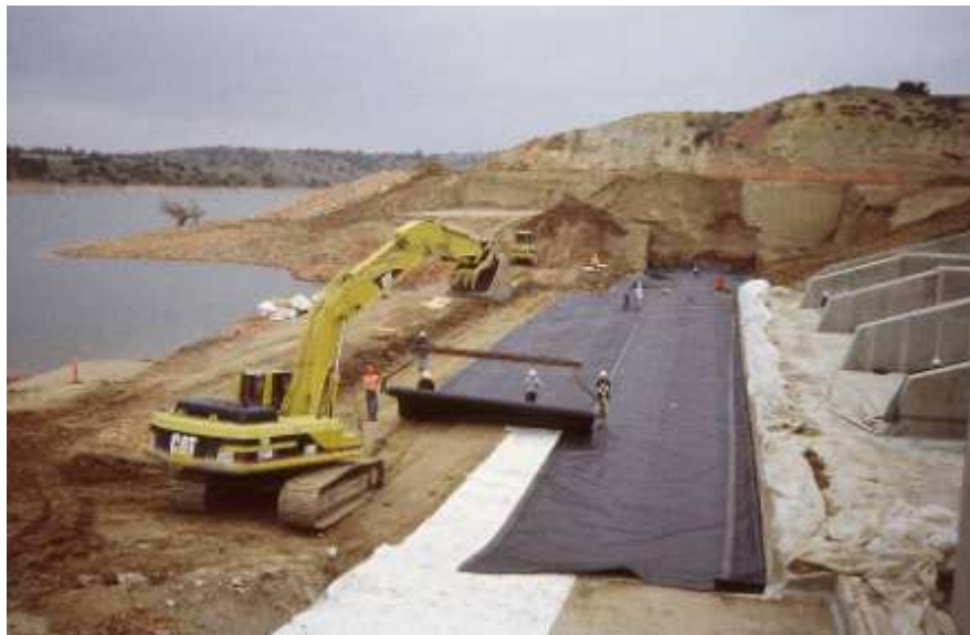
Photograph 7.13: Geosynthetic clay liner and geomembrane liner being installed as remedial seepage barriers upstream from a new spillway at Tongue River Dam, Montana USA. The horizontal geosynthetic barriers were connected to the concrete spillway slab and to a deep vertical sheet pile seepage barrier in front of the spillway (Miller et al., 2001)
