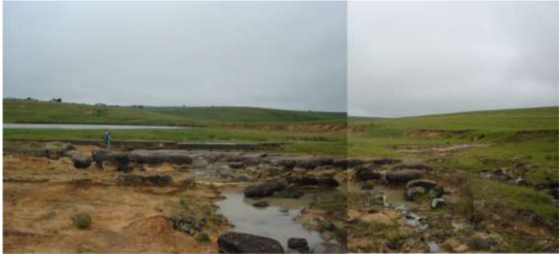
Photograph 7 .1: Backward erosion of the by-wash Spillway of Toleni Dam in South Africa
