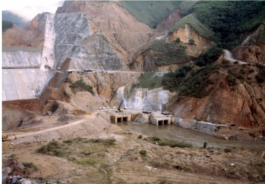
Figure 7.1- Residual Soils Found at the Right Abutment (Far Left) at Salvajina Dam that mandated special treatments at the Plinth and Foundation.
