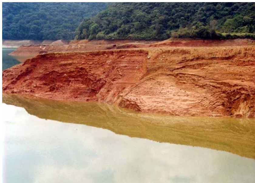
Figure 8.3- Reservoir's Slope Instabilities Experienced at Punchiná Dam Due to Rapid Drawdown (INGETEC S.A., 2002)
