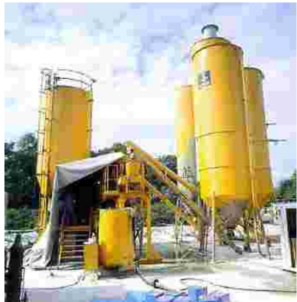
Fig. 4 Stationary slurry batching and mixing plant
