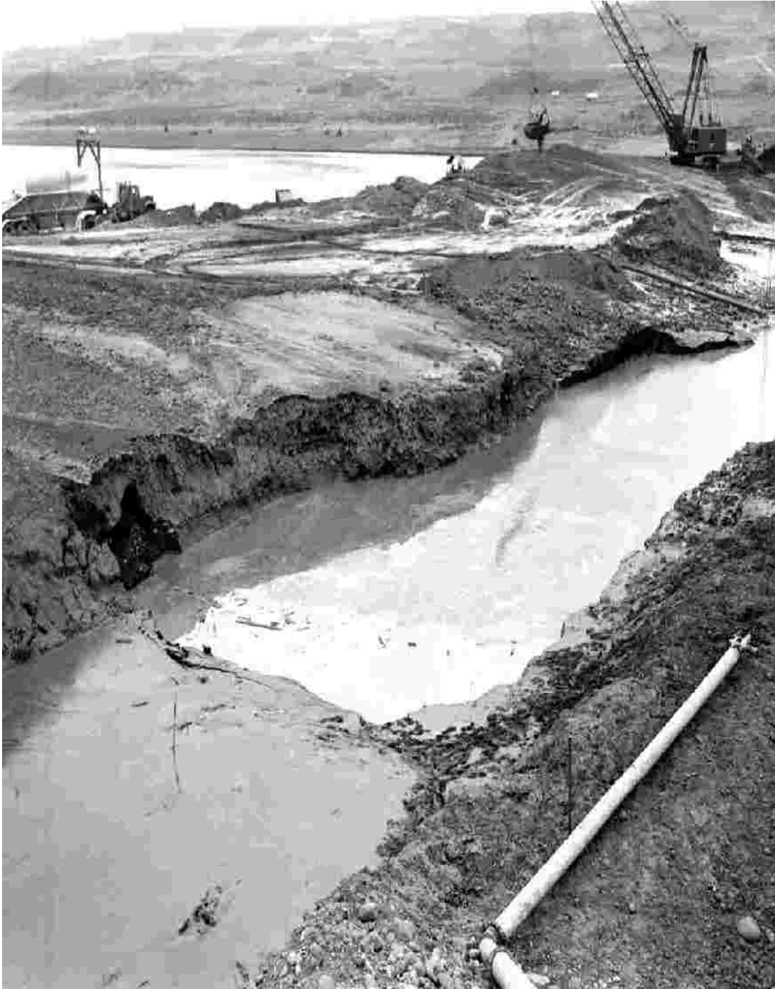
Figure 4 Slumped slurry trench
