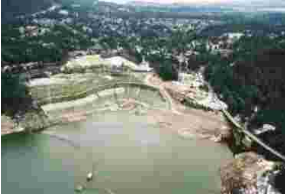
Fig. 3 Aerial view of the seepage control work on left abutment. Cleveland dam is at the lower right hand corner.
