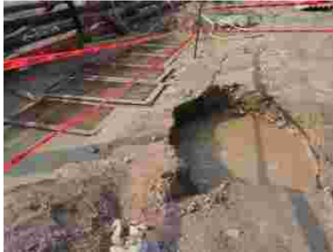
Fig. 11 Sinkhole near the open trench
