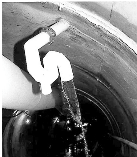
Fig. 7.15 – Siphon in a dam foundation gallery in order to avoid that the leaking water from a limestone formation is exposed to carbon dioxide of the air.
