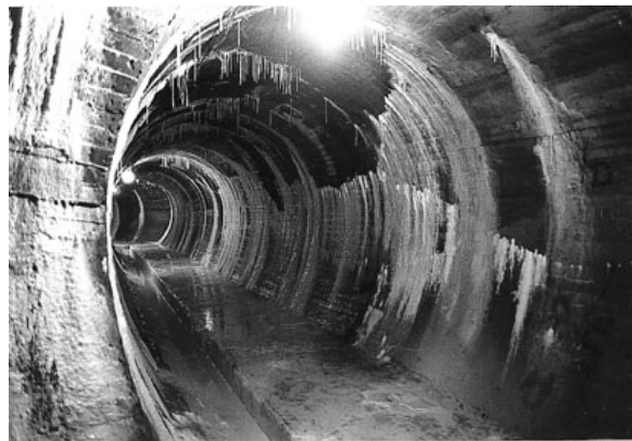
Fig. 7.16 – Excessive deposit of \text{CaCO}_3 - leaching from cement grout - in a dam foundation gallery.
