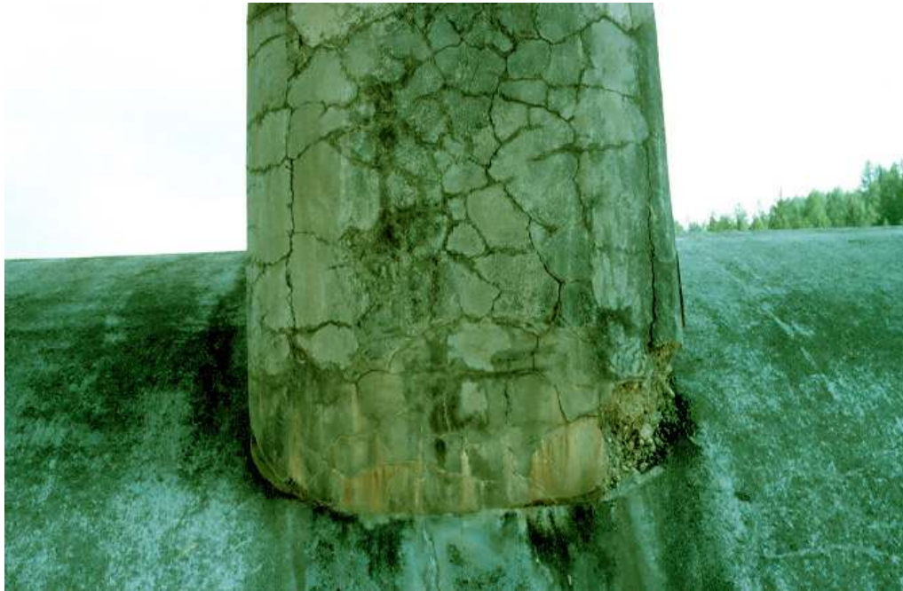
Fig. 8.2 - Concrete spalling on a spillway pier [8.3]
