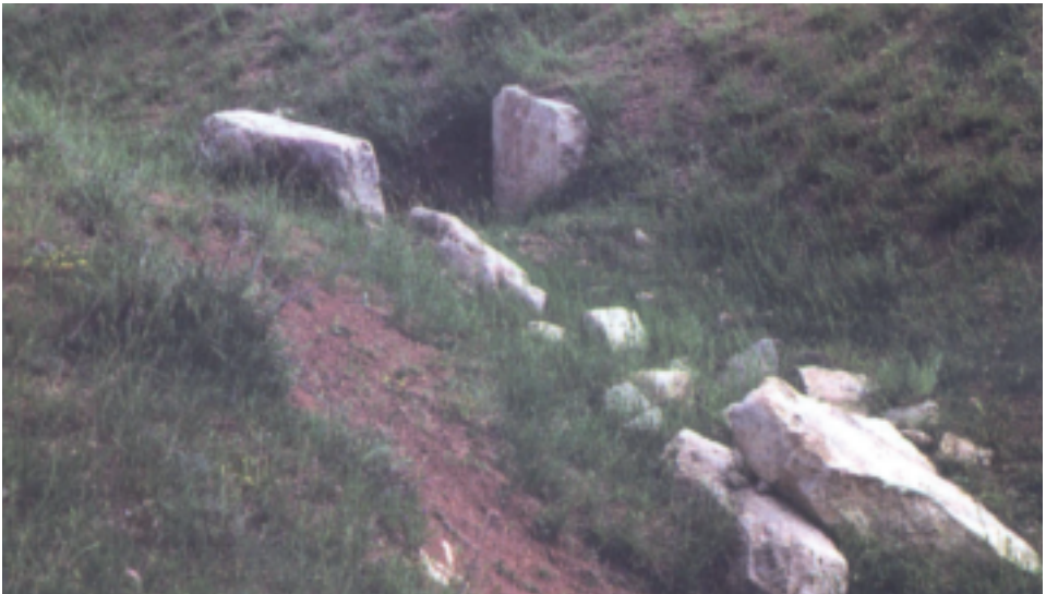
Fig. 71 Remains of the bottom outlet of Karakuyu dam before excavations
