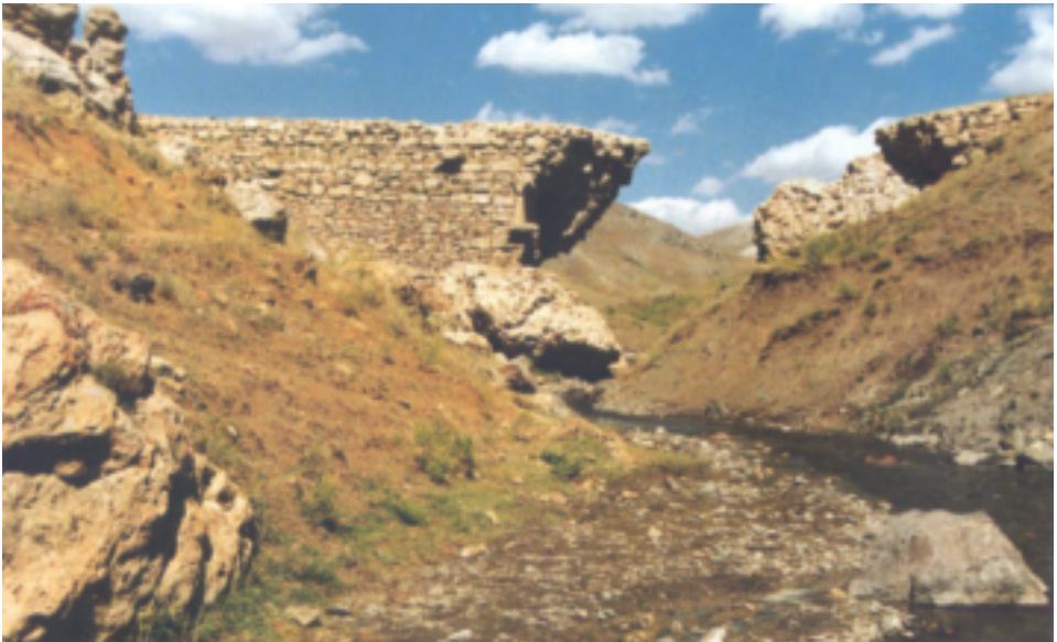
Fig. 79 Faruk dam, after the collapse of the left abutment half
