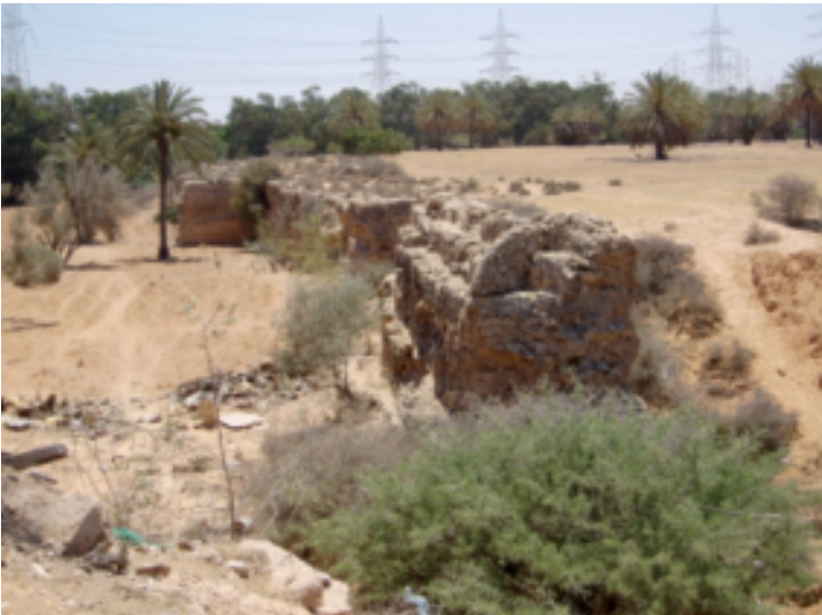
Fig. 47 General view of Old Libda dam from the left abutment, with 5 m of maximum height and 200 m long
