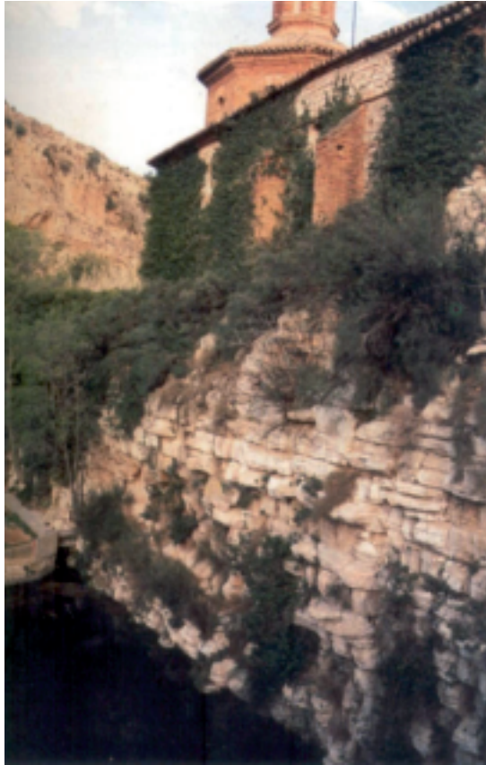
Fig. 60 The Roman Dam of Muel from downstream with the 18th-century hermitage constructed on top (Arenillas/2006)
