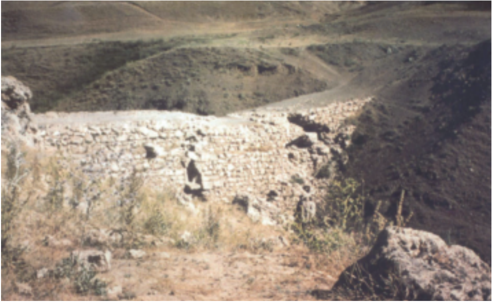
Fig. 78 Downstream view of the 12 m high Faruk dam, with 30 m crest length (left abutment half of it, to the right-hand side of the picture, collapsed in 1988) near Van
