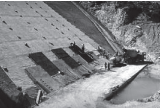
Fig. 65 Bovilla dam, Albania 1996, new construction: unreinforced concrete slabs are cast in situ over a geotextile protecting the PVC geocomposite from concreting
