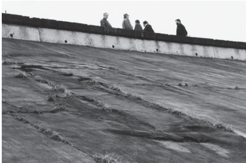
Fig. 36 Growth of vegetation on bituminous geomembrane (ultimate condition)
