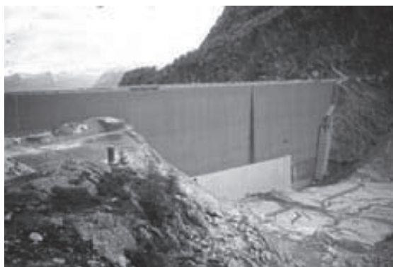
Fig. 75 Alpe Gera, Italy 1993, 174 m high. A 2 mm thick PVC geocomposite waterproofs a 3 mm thick deteriorated steel lining
