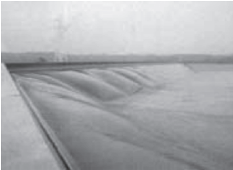
Fig. 30 Okinawa reservoir, Japan. Effect of wind uplift on an exposed geomembrane anchored by continuous lines. Photo taken during a typhoon, wind velocity > 175 km/h
