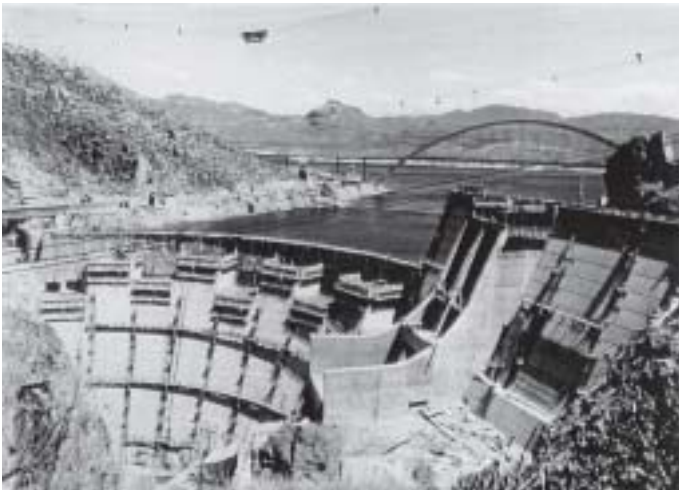
Fig. 6.36. Photograph taken during modifications of Theodore Roosevelt dam Photo prise pendant les modifications au barrage Theodore Roosevelt
