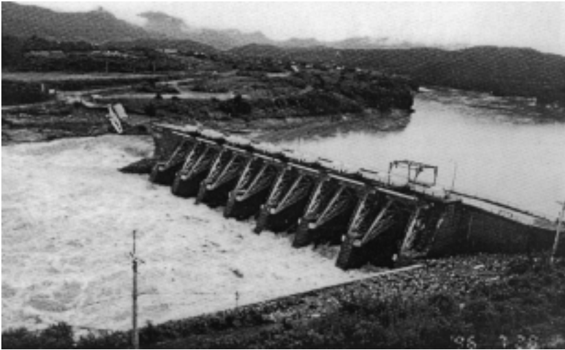
Fig. 3.21 The failure of Yeon-cheon dam
