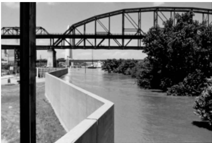
Fig. 5.20 Floodwall at St. Louis, Missouri. Mississippi River looking upstream at St. Louis (Photo courtesy of U.S. Army Corps of Engineers)
